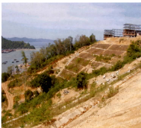
Hill cutting and construction activities degraded the coral reefs near this site
